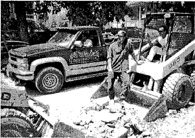
Workers for Swain Construction Inc. are making good progress, shown here moving the last pile of concrete near 31st and Chicago Streets.
